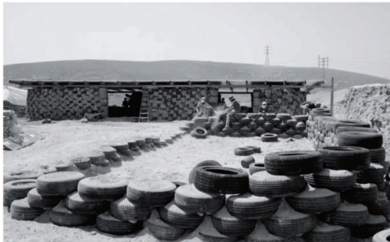
Costruzione della scuola a Khan al Abmar, Territorio Occupato Palestinese, 2009. Tecnica Earthship. / Construction of the School in Khan al Abmar, Occupied Palestinian Territory, 2009. Earthship Technique.
