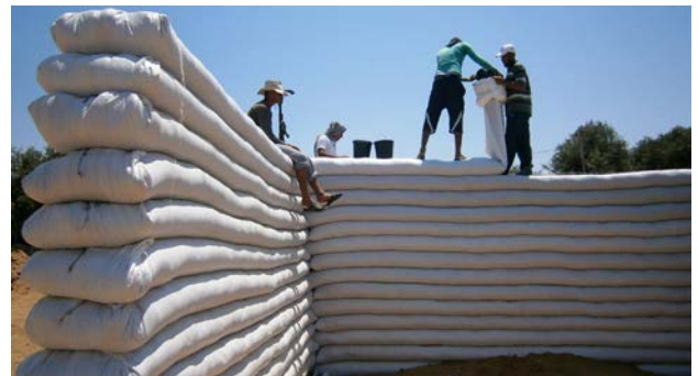
Fig. 2: Construction of earth-bag walls for Um al Nasser children's center. Design by: ARCò, & MCA. Promoted by: Vento di Terra ONG.
