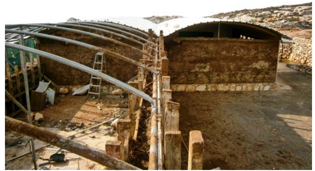
Fig. 4: Ramadin al Janub's school being upgraded from temporary to permanent structure using rammed-earth technique. Design by: ARCò. Promoted by: Vento di Terra ONG.
